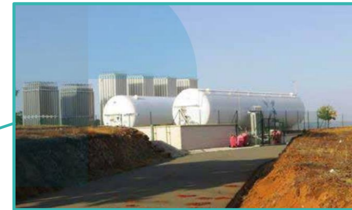
Mainly Autonomous Natural Gas Regasification Units (UAG)
