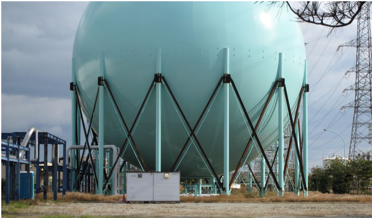
Figure 13. Additional bracings to reinforce the support legs of a spherical storage tank against earthquakes.
