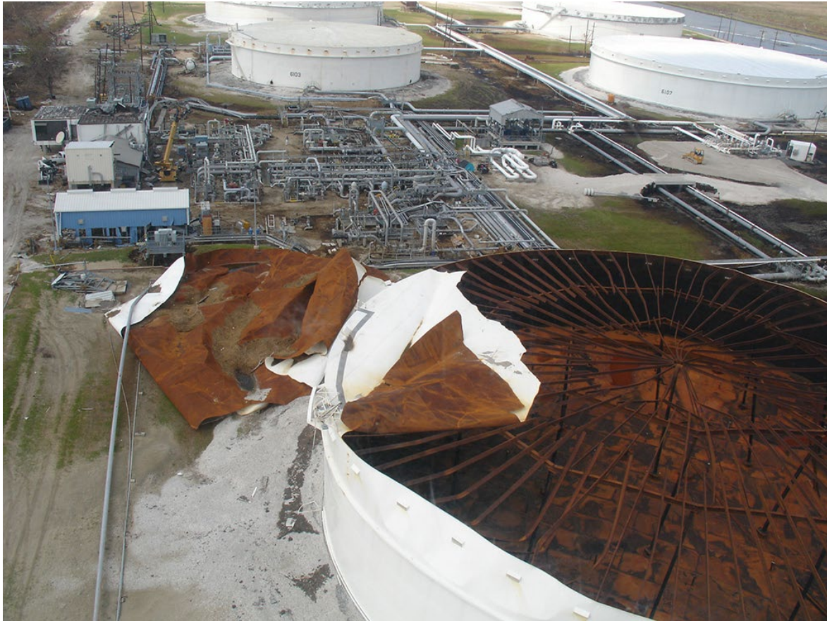
Figure 8. Damage to the fixed roof of an atmospheric storage tank caused by strong wind.
