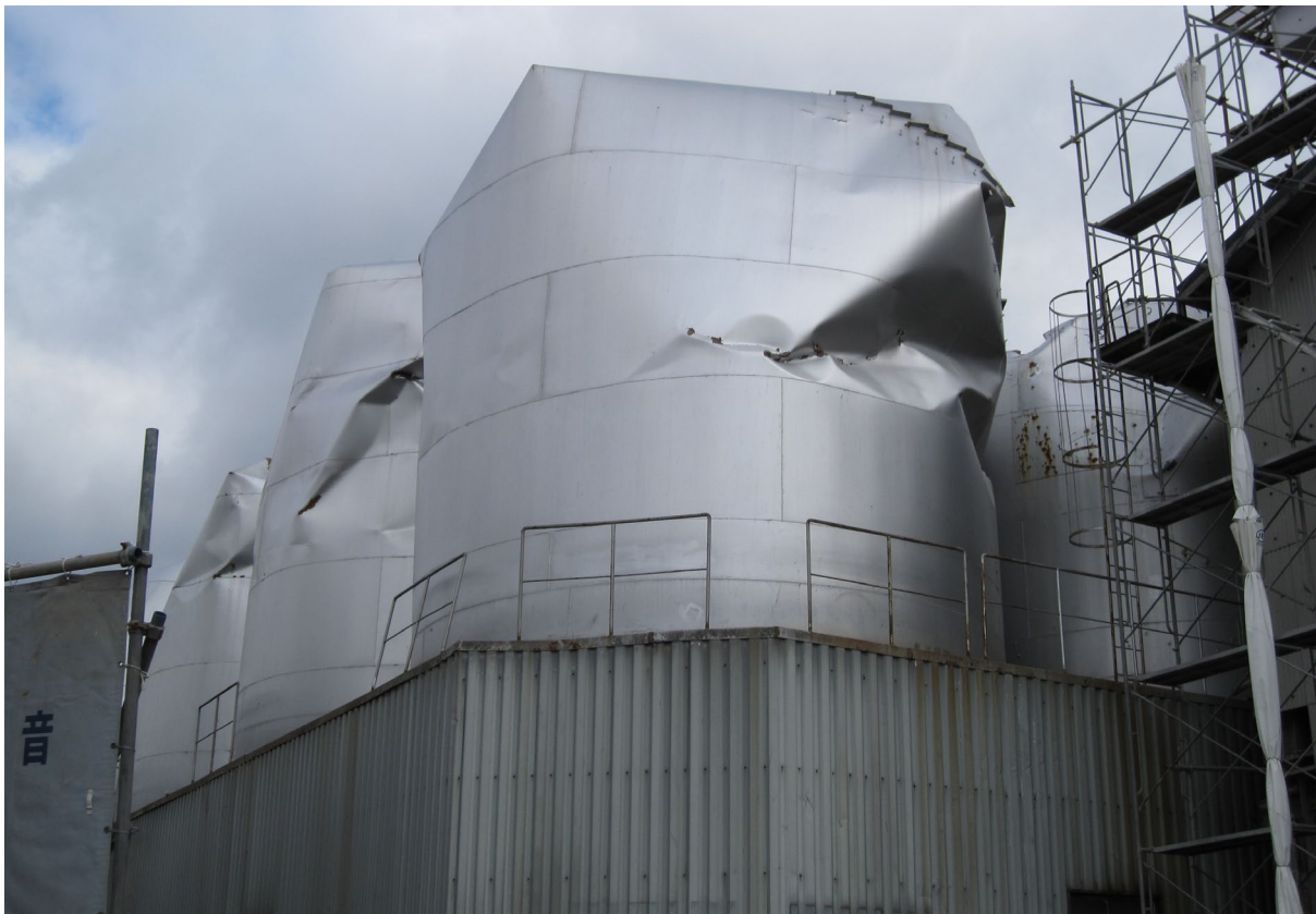
Figure 4. Buckling damage due to an earthquake at silos.
