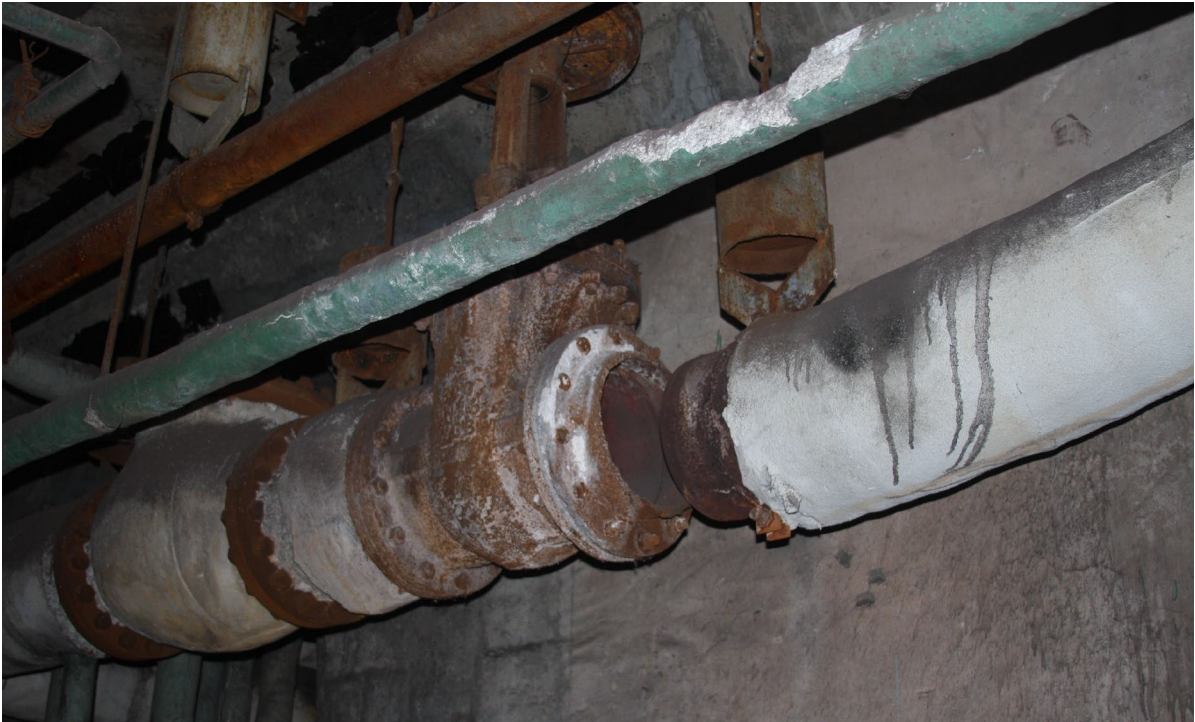
Figure 5. Pipe break at flange connection during an earthquake.
