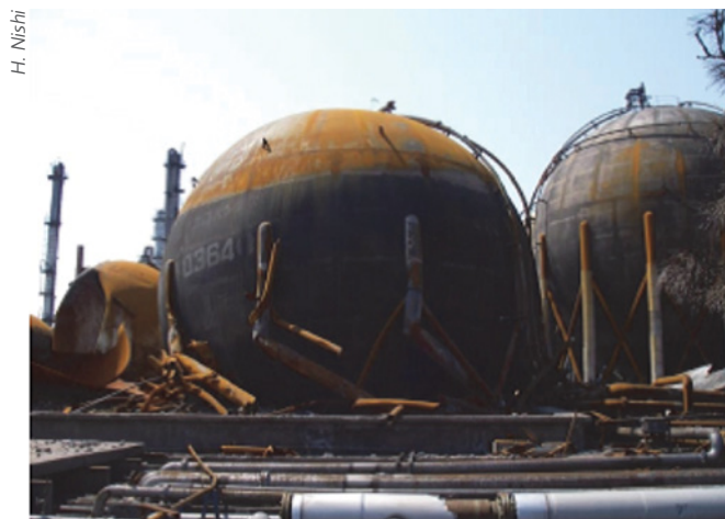
Figure 2 – Buckling of tank legs due to earthquake
