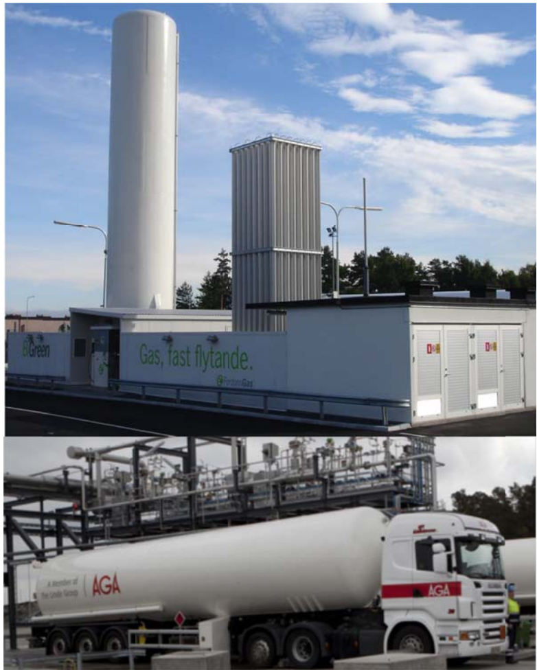
Figure 5 A typical PLNG gas supply for an industrial facility (C. Sandqvist, MJV Workshop [2])
