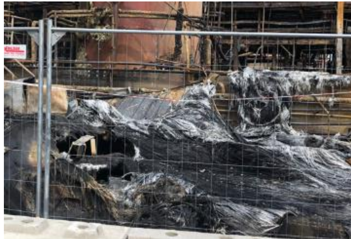
Collapsed Fiberglass tank
