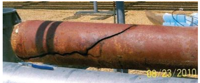
Figure 2. Ruptured 12-inch diameter end cap of low-temperature suction line piping on the roof of the facility.
