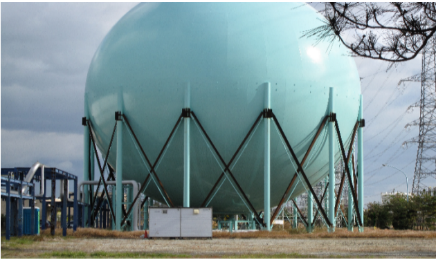
Figure 2. The bracing system of this LPG tank was reinforced after the 2011 Great East Japan earthquake and tsunami (Photo credit: E. Krausmann)
