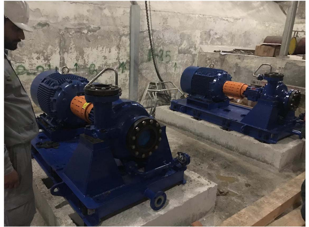
New Blue Pump Room
