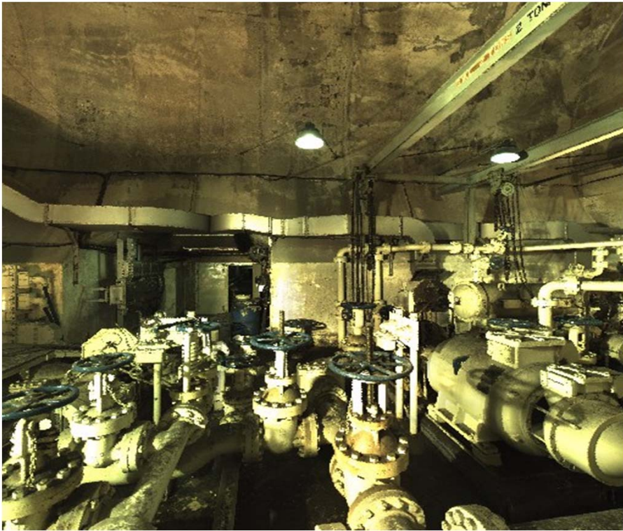
Existing Blue Pump Room
