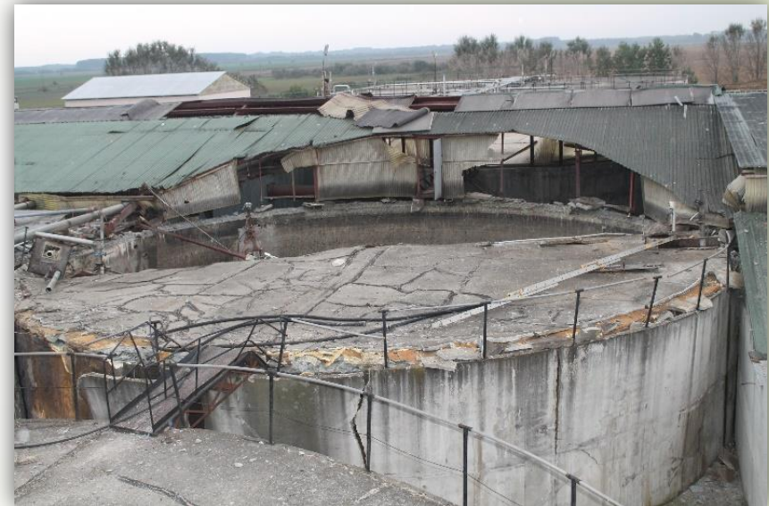
October 2021. Digester explosion Biogas plant 3 victims (subcontractors)
