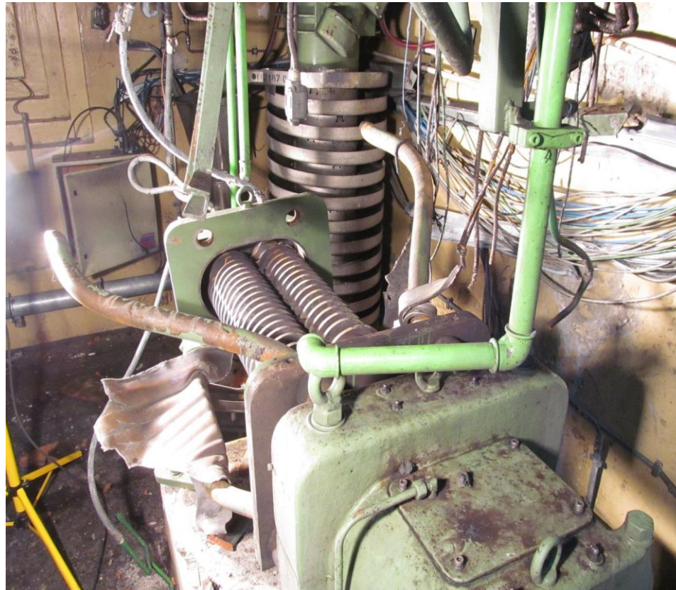
inside view box, kneader and housing devastated
