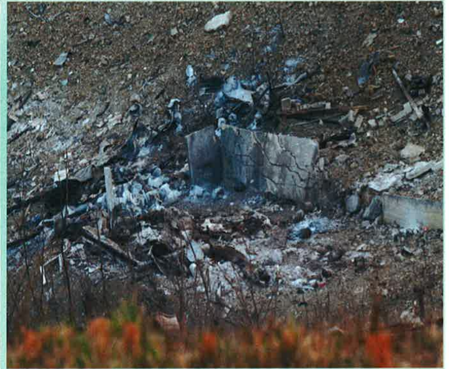
Damages caused to the buildings and their protection walls
